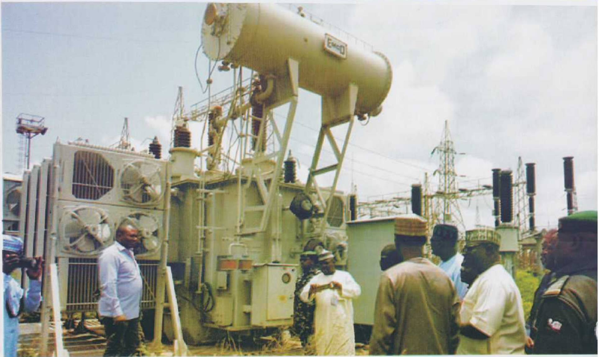
The newly acquired Transformer for improved power supply in Zamfara
