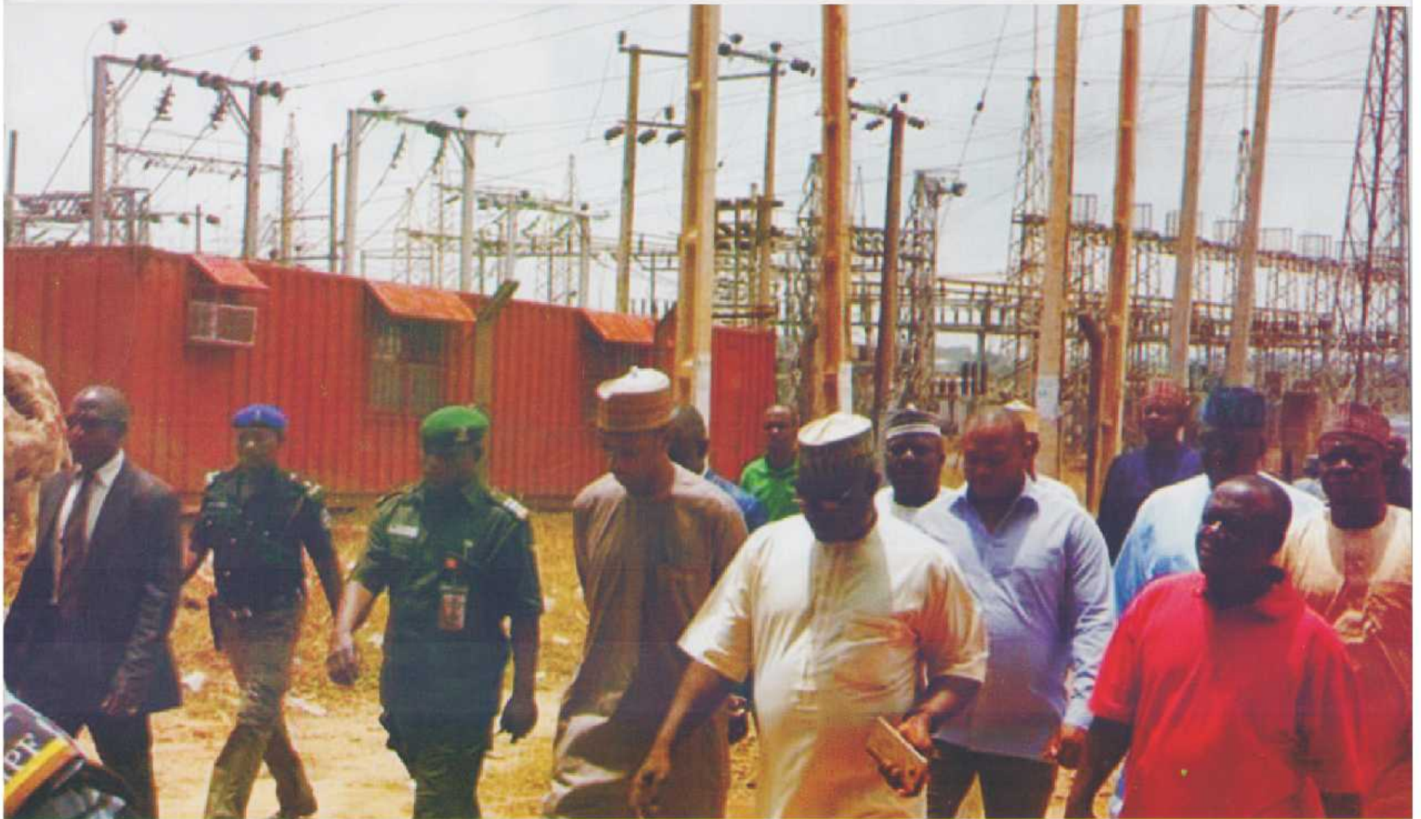
His Excellency Deputy Governor at the Commissioning of the new Transformer
